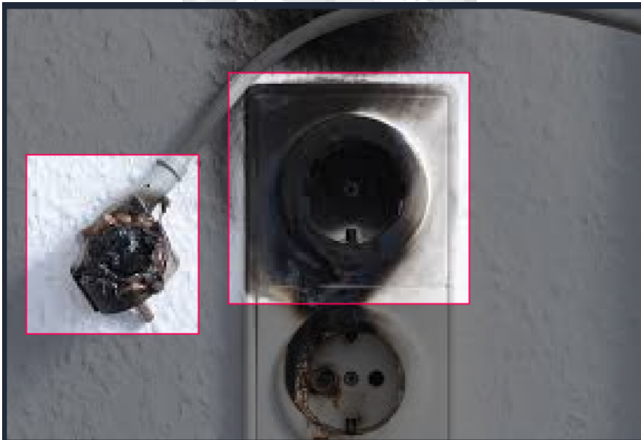
Figure 3.3: Electrical hazard image used for training, hazard enclosed by red bounding box
