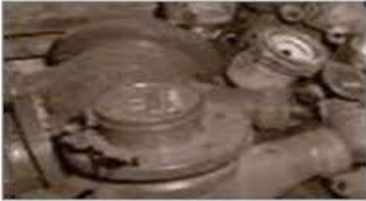
Water meter damaged from frost
